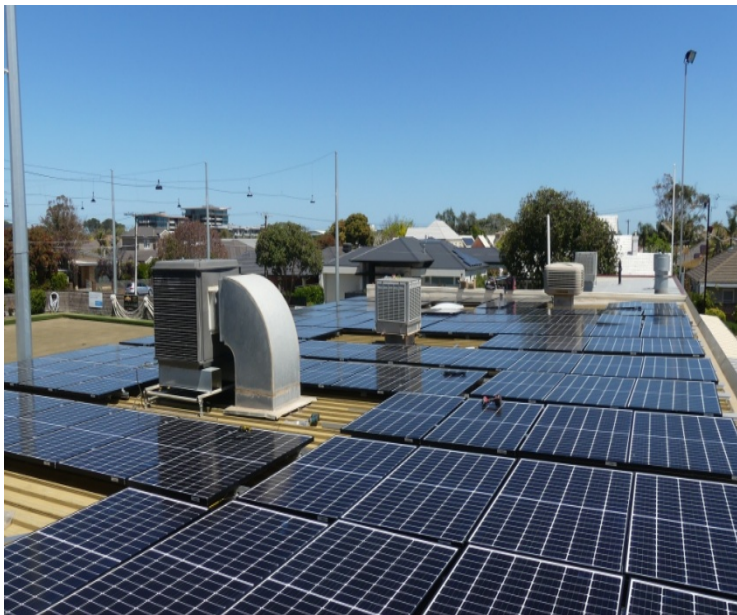
Solar Panels on the roof busily producing electricity.
