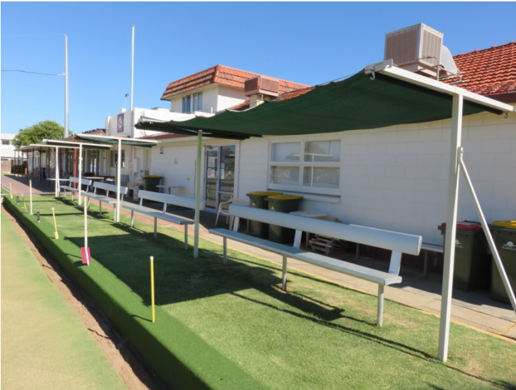
New shade cloth shelters erected on the north border of A green.
